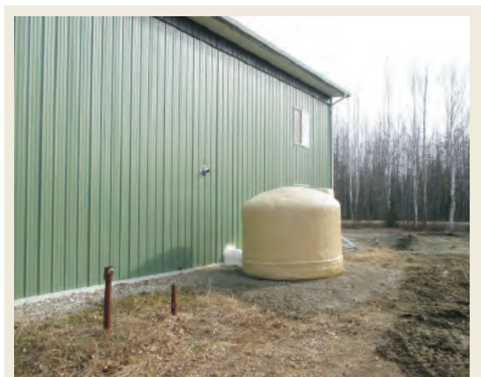
Above Ground Water Tank
